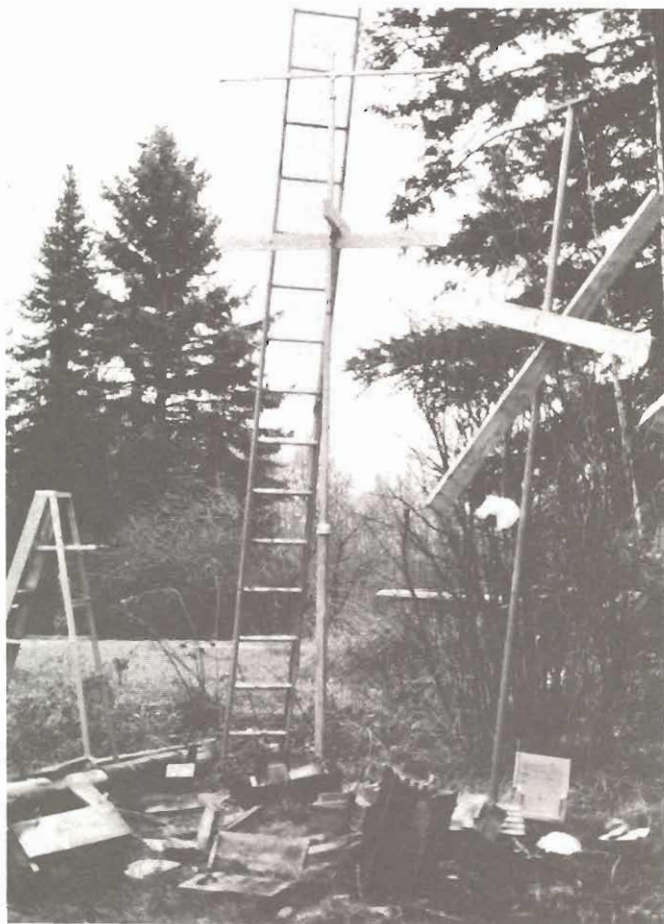
Destruction of remaining feeders on pole at right. New pole erected on left with lowest crosspiece at 10 feet. Step ladder shown is 6 feet high.
